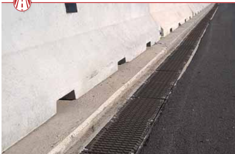
National Road S.S. Sassari - Olbia Drainage channels (Sardinia, Italy)
